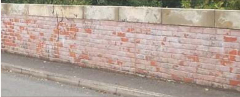
Unsuccessful anti-graffiti coating
